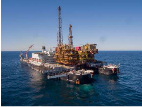
The Allseas Heavy Lift Vessel Pioneering Spirit lifting the topsides of a platform on a previous project
