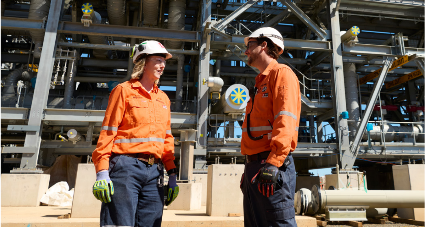
Woodside CEO and Managing Director Meg O'Neill said 2024 was a year of significant progress at the Pluto Train 2 site, with all 51 modules arriving safely and being set by year end
